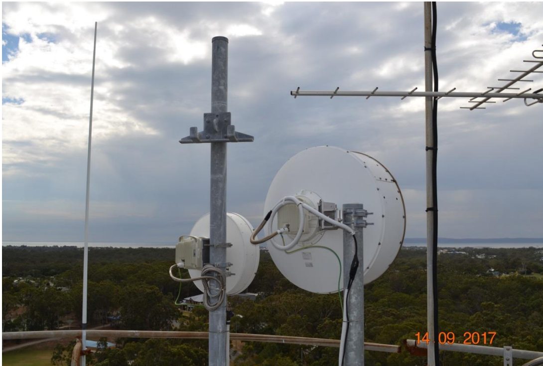
Photograph No. 2 - Safety barrier rail in poor condition on the roof of the Alexandra Hills High Level Reservoir Tower showing complete dislodgment in right hand bottom corner
